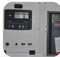
Control Panel & MCB
